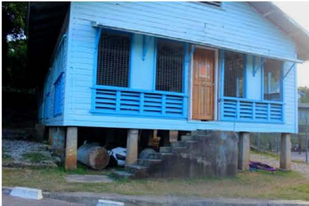
House on stilts, posing difficulties for people with mobility issues during emergencies
